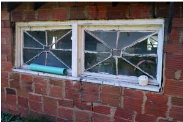
Windows once installed in the main Dance Pavilion. They were removed by a worker after one of the major fires which occurred after the park permanently closed. After being stored for a couple years, they were then used in the construction of this garage in 1915. The garage, originally built as a laundry room, still stands in the Park Gate area.
