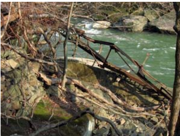
Another view of the wreckage of the upper bridge.
